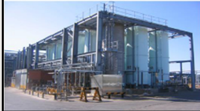
STORAGE & TANK FARM
